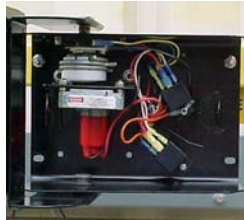
7. Inside view of control box.
