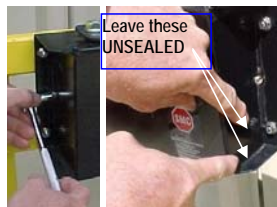
30. Re-install screws at both ends. Re-seal w/black silicone leaving bottom & 1/2" on bottom side open for drainage.
